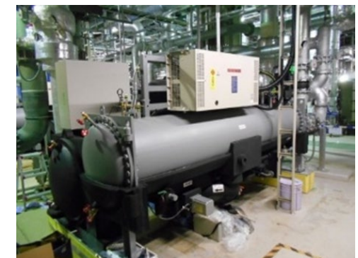
Centrifugal chiller with new refrigerant
