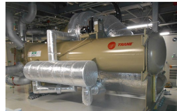
Centrifugal chiller with Non-Freon refrigerant
